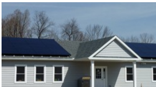
Solar panels on the Town of Caroline Office Building
